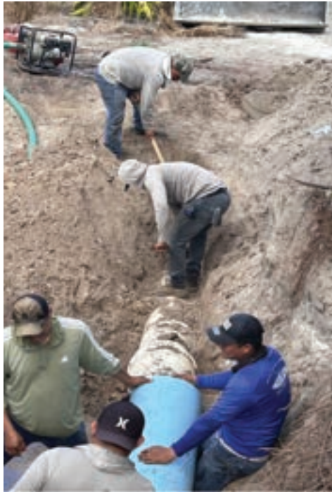
▲ Another 16-inch mainline break in 2024 that was about 25 yards from the 2023 break in the previous pictures.
