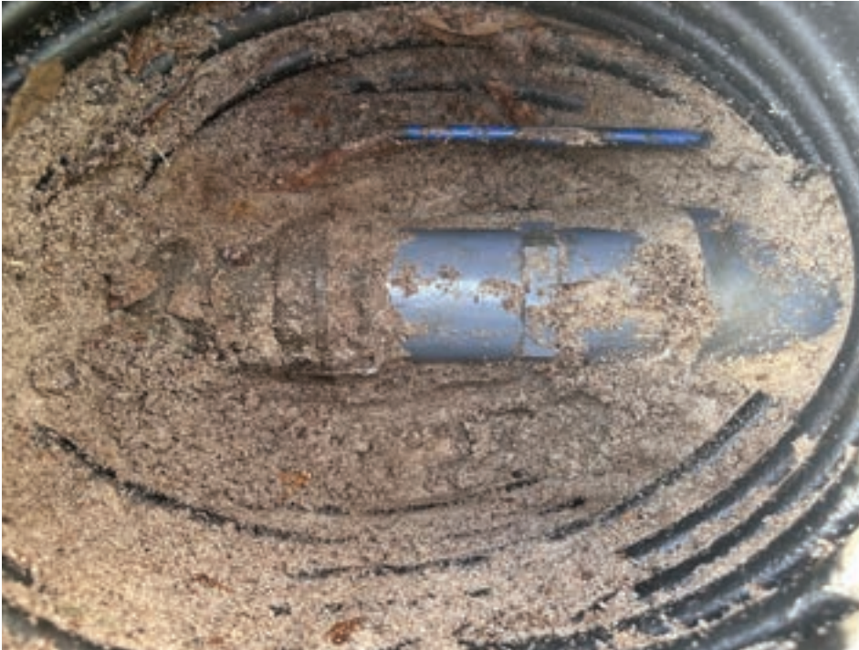
▲ Another lateral water line valve with a collapsing box and a handle broken off due to rust/corrosion. This problem exists in about 80% of the lateral irrigation valves.
