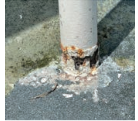
▲ Rusted canopy poles throughout
