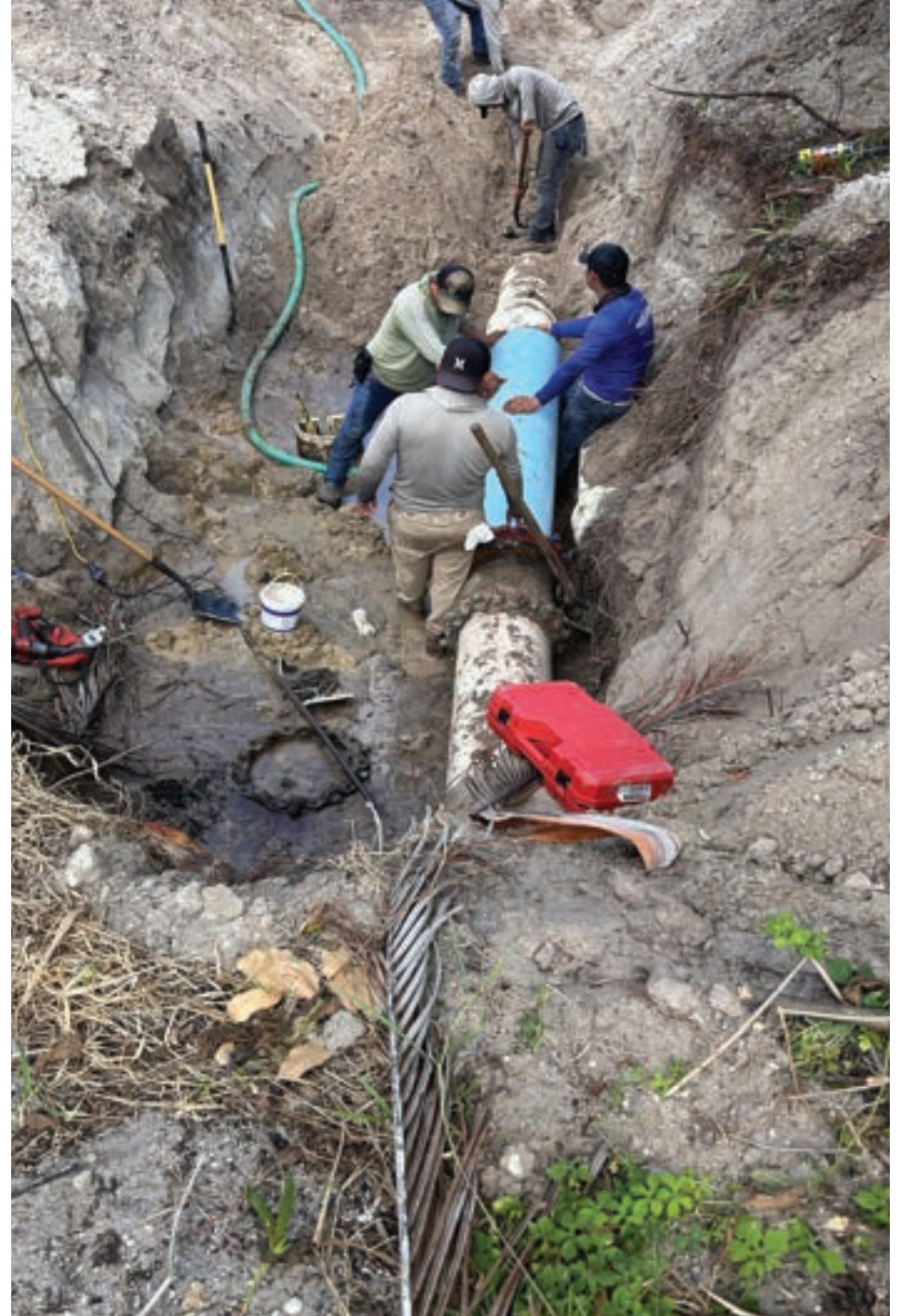
▲ 16-inch mainline break in 2024. We must call an outside company for these repairs as we do not have the tools for this application. 16-inch mainlines are rare in today's irrigation designs for this reason.
