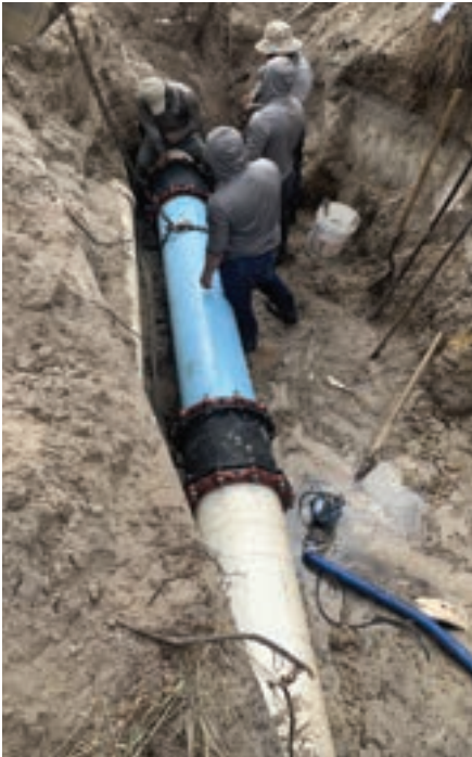
▲ 16-inch mainline break in 2023.
