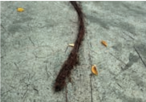
▲ Roots pulled from watering system pipes
