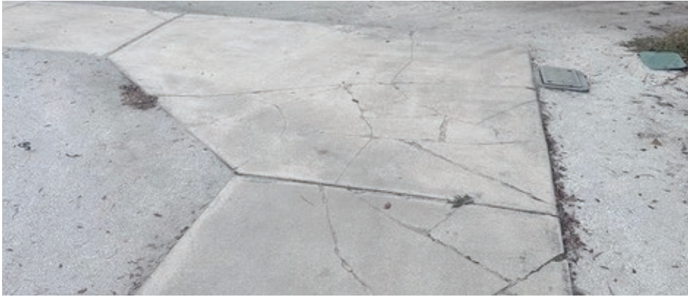
▲ Cracked sidewalks presenting safety issues
