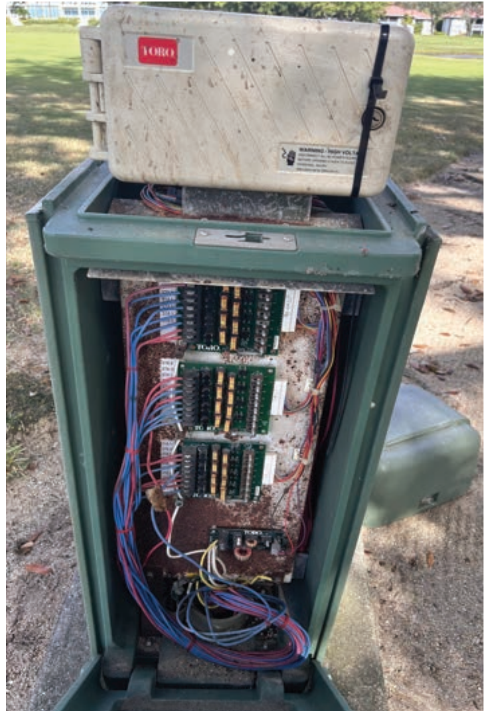
▲ All the tops of the electronic control boxes are being held with zip ties. Rust and corrosion exist throughout all the boxes as well. The front 9 is wired for 110V and the back 9 is wired for 220V.
