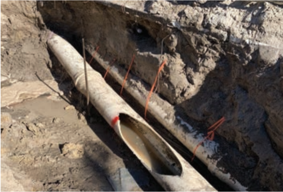
▲ 16-inch water mainline break in 2023.
