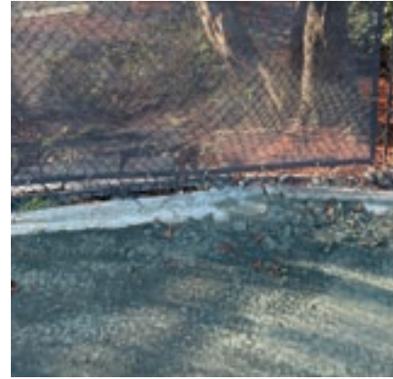
▲ Edge of court lifted due to root growth
